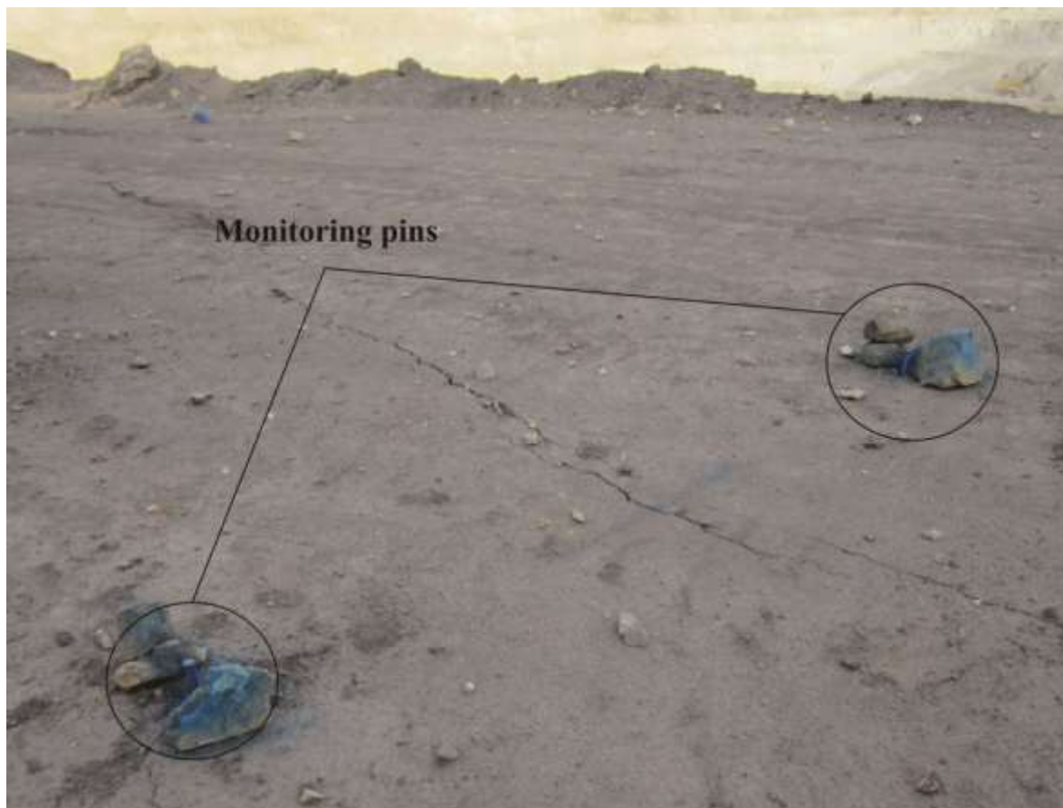
Figure 5. The installed monitoring pins to monitor the displacements around the F-a fault hanging wall on top of the slope under study. Tension cracks are observed around these pins.
