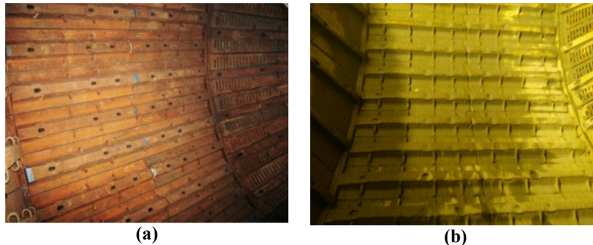
Figure 6. (a) The original and (b) new liners installed in the SAG mill of phase 2.
