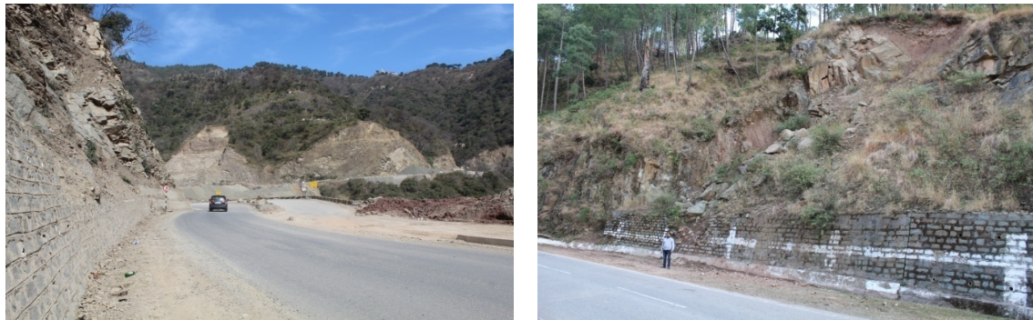
Figure 1 Poor performance of retaining walls in the Himalayan region, especially where road construction is ongoing
